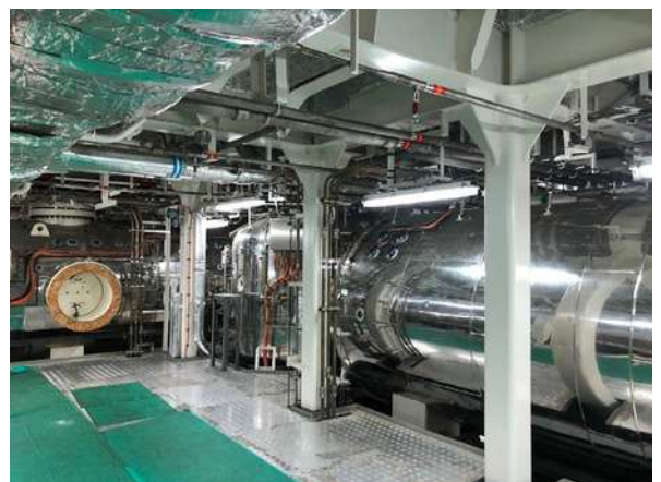
Saturation Diving Chambers
